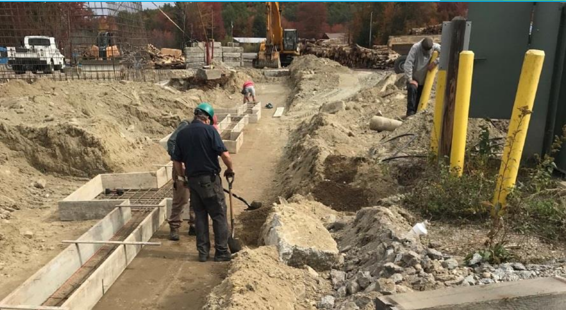
Excavating on an Expired Dig Safe Ticket
