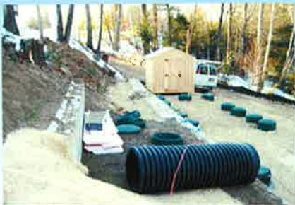
AFTER THE 3 BIOCON TANKS WERE SET, THE FIRST TANK FARM AREA IS NEARLY DONE-LOTSA RISERS
