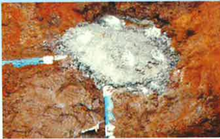
AFTER ETTI PULLED IN A 200 PSI 2" LINE A SWEEP AND TRUST BLOCK CONNECTION WAS MADE
