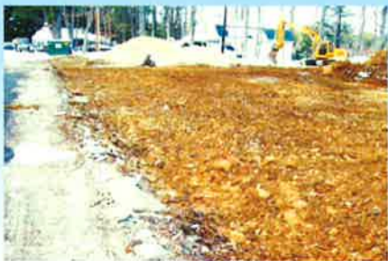
LEFT A LOOSE SURFACE WITH STILL SOME CHUNKS-SAND STAGED IN FOR SPREAD AFTER INSPECTION
