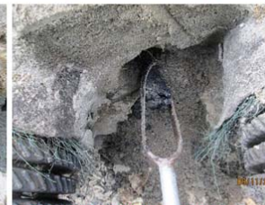
End Opposite from Inlet Between Rows #3 & #4 Showing Black Anaerobic Sand at 1 FT Depth
