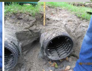
End Opposite from Inlet at Row #8 Shows Insufficient System Sand & Cover Over Pipes
