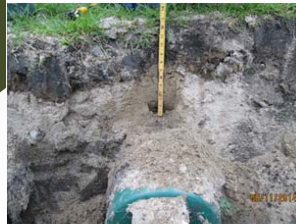
Inlet End at Row #1 Shows Correct Amount of System Sand Over Pipes
