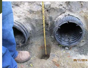
End Opposite from Inlet Between Rows #2 & #3 Showing Plenty of System Sand Under the Pipes
