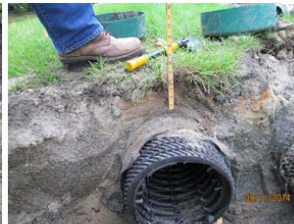
Inlet End at Row #8 Shows Insufficient System Sand & Cover Over Pipes
