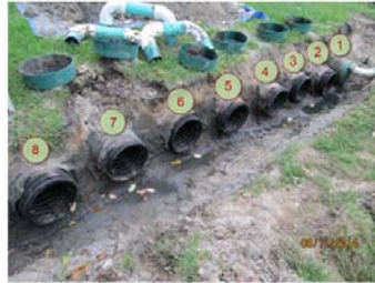
Inlet End of System Showing Order of Effluent Flow
