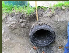
End Opposite from Inlet at Row #1 Shows Insufficient Amount of System Sand Over Pipes
