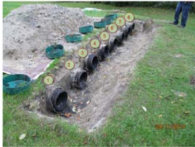
End Opposite from Inlet Showing Order of Effluent Flow
