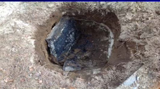
Totally clogged d box result of missing outlet in tank for 6 years
