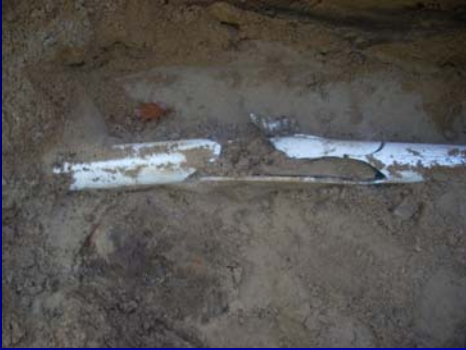
Improperly bedded pipe
