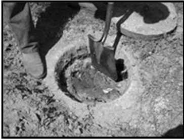
Neglected septic tank, never pumped. The contents of sre hard enough to walk on. The tank had to be abandoned and an entirely new tank and septic field had to be installed.
