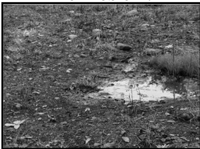
Grease clogged drain fields make it impossible for soil to absorb and treat liquids. May require a new drain field.
