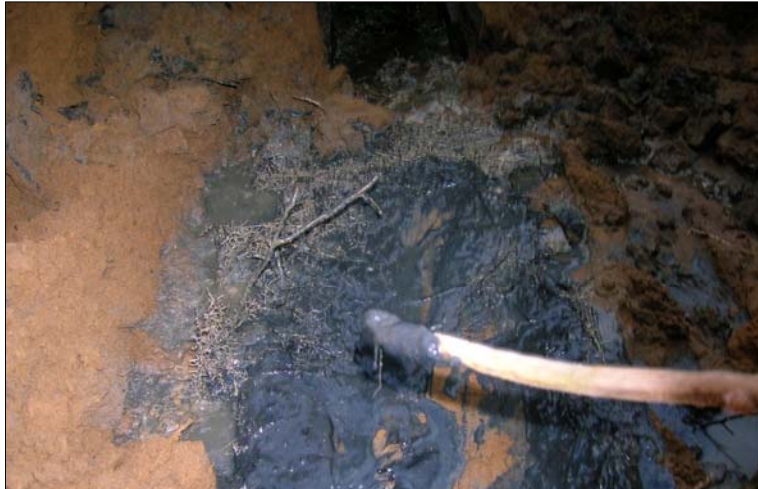
Oily slime was discharged to this drainfield, clogging the infiltrative surface and causing malfunction
